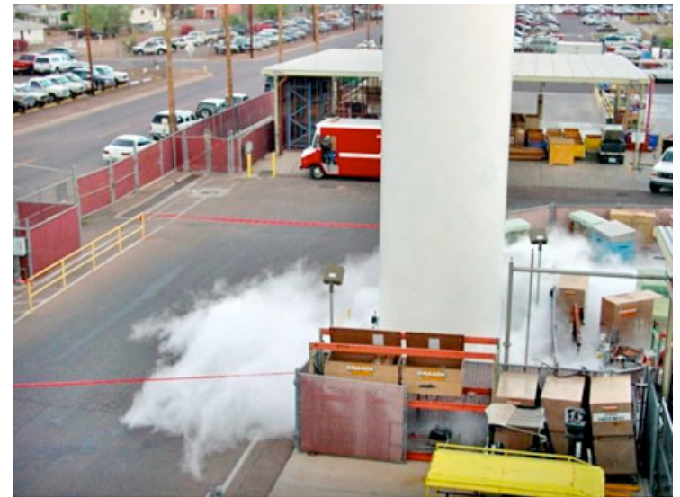
A liquid hydrogen release will look similar to this liquid nitrogen release. (Photo courtesy of Scott Stookey)
