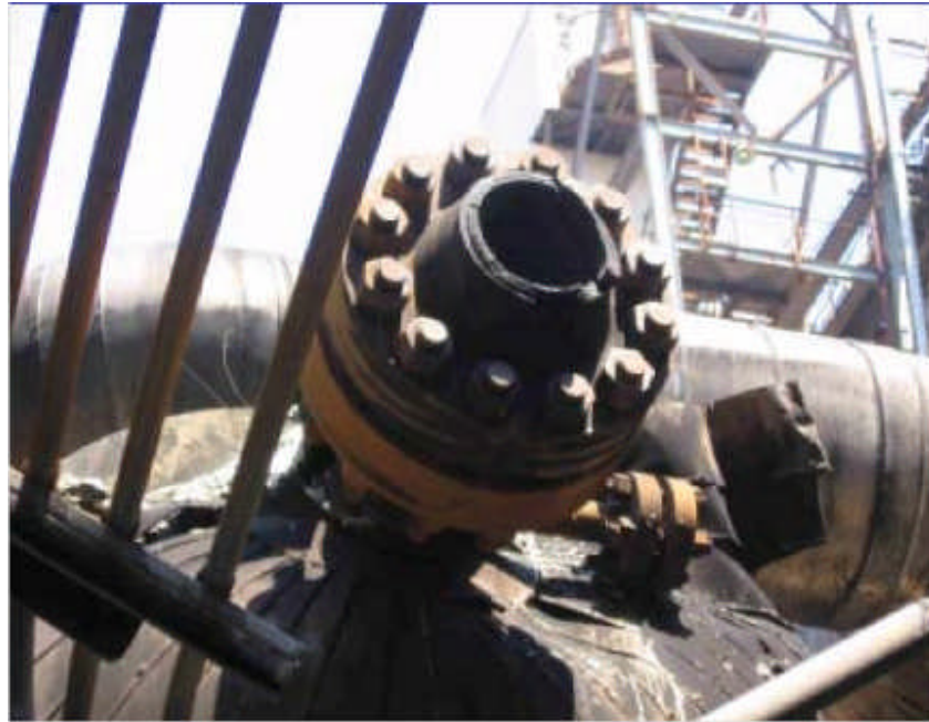
Figure 3. Ruptured 8-inch pipe elbow on heat exchanger A outlet
