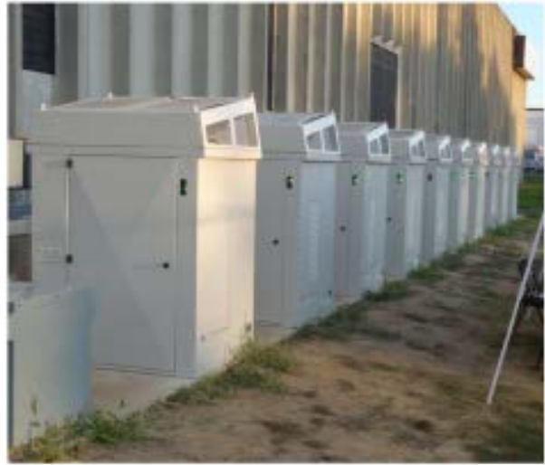
Figure 4. Packaged Fuel Cell Units Providing Stationary Backup Power
