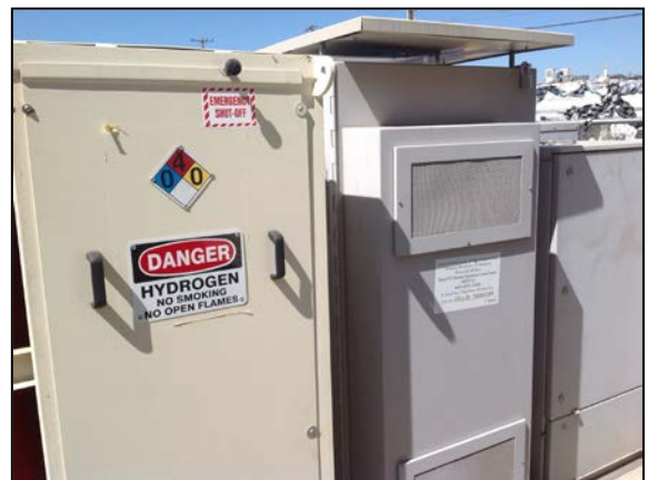
Figure 5. Bulk Hydrogen Storage Containers
