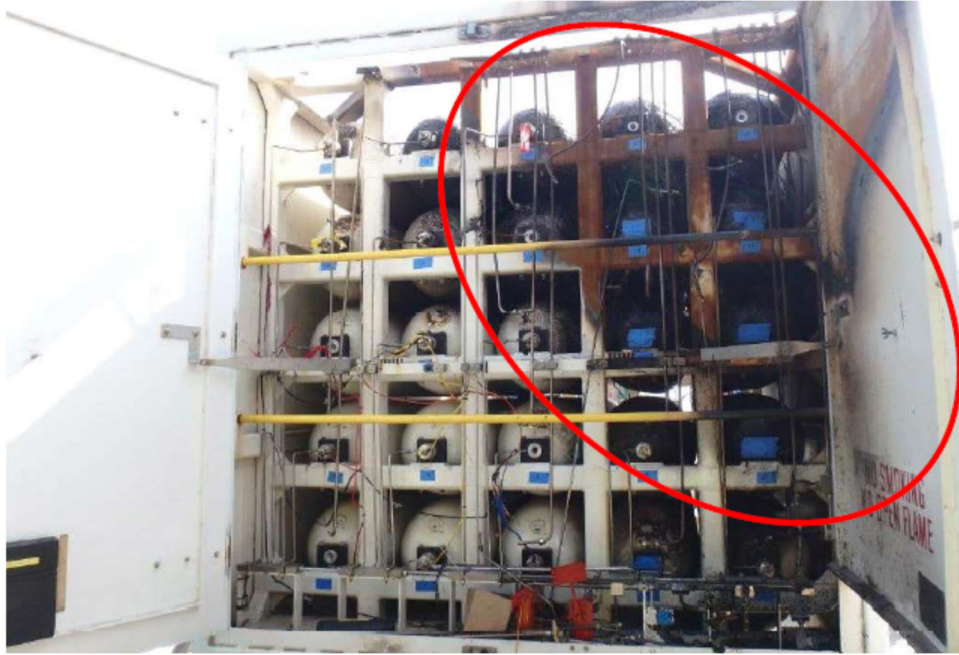
Figure 2. Cylinder ends in open incident trailer with fire-damaged cylinders encircled (from NTSB report)
