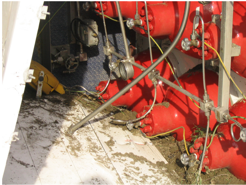
Figure 3° Breakup valves of head of the cylinders of the wagon
