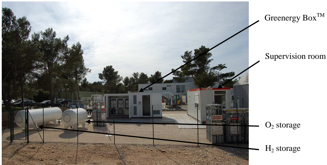
Figure 3: Greenergy Box™ settlement on HELION's site.
