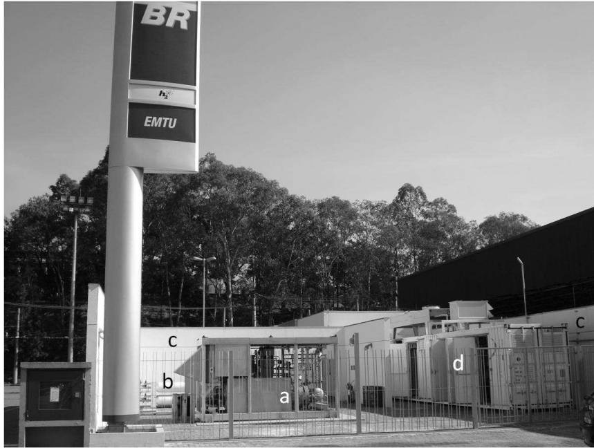
Figure 2: View of the back of the Hydrogen Fueling Station: a) compressor; b) hydrogen storage cylinders; c) fireproof walls; d) container with the alkaline water electrolysis system.
