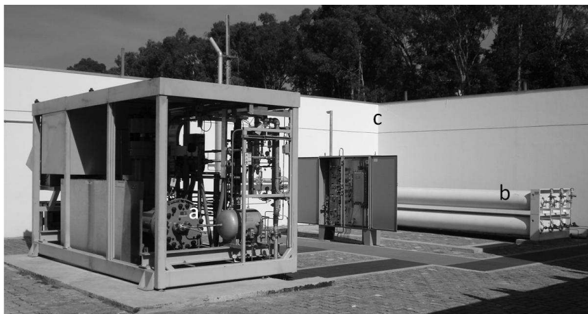
Figure 3: View of the back of the Hydrogen Fueling Station: a) compressor; b) hydrogen storage cylinders; d) fireproof walls.
