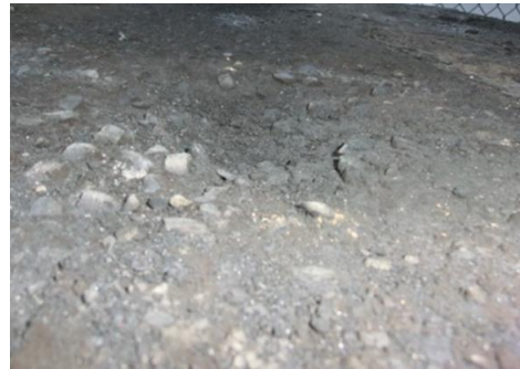
Fig.2 Burnout traces on asphalt road
