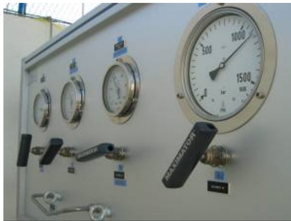
Figure 9 – High pressure manifold
