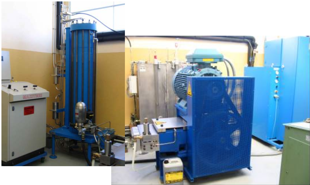
Figure 1: General view of hydraulic machines
