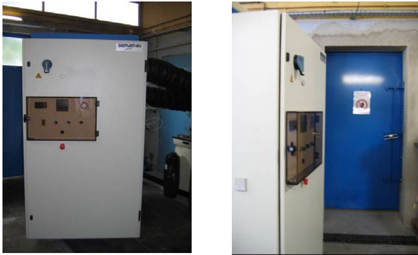
Figure 5. Air generator and bunker
