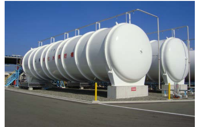
Liquid hydrogen storage tank
