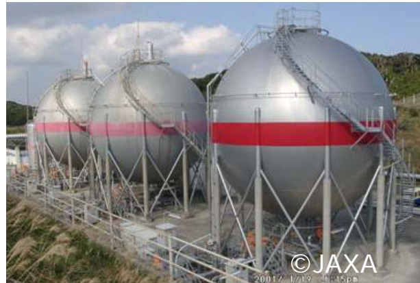
H-II rocket fuel hydrogen storage tank
