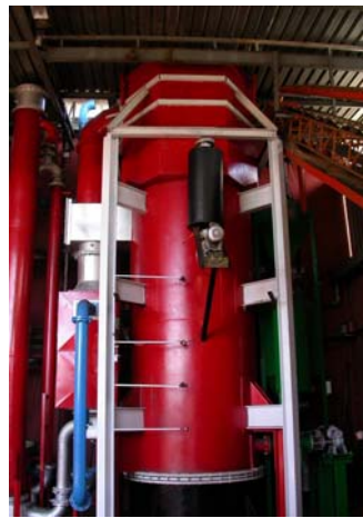
Figure 1. Bubbling fluid bed gasifier (courtesy of EQTEC Iberia, S.L. and Energía Natural de Móra, S.L.).
