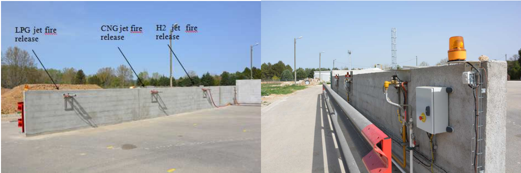
Figure 7. Operational jet fire platform (left) and its technical area protected behind the wall (right).
