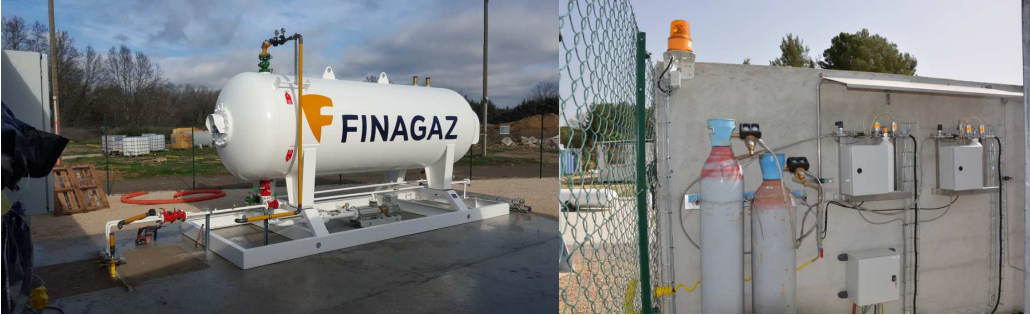
Figure 6. LPG storage (left) and technical installation for the explosion platform (right).
