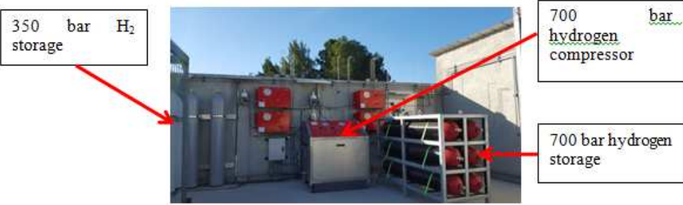
Figure 5. Hydrogen 700 bar compressor and 700 bar storage of the technical platform.
