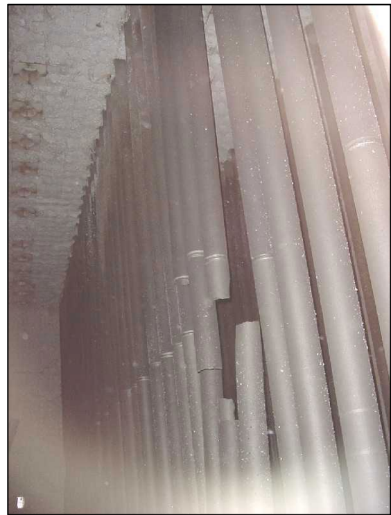
Figure 1. Tube failure from thermal shock
